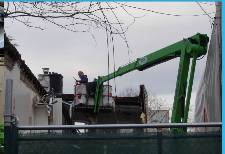
1846 New York Avenue, Brooklyn. Explosion in cellar.
