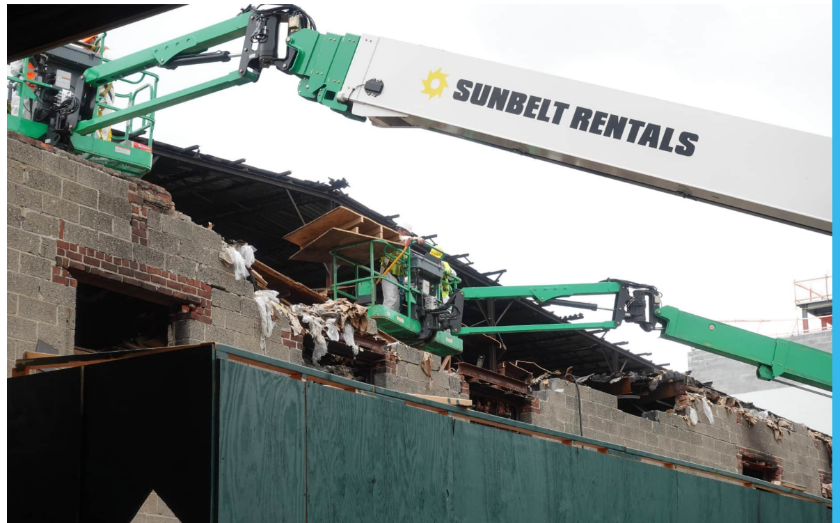
259 Monitor Street, Brooklyn. Fire damage.
