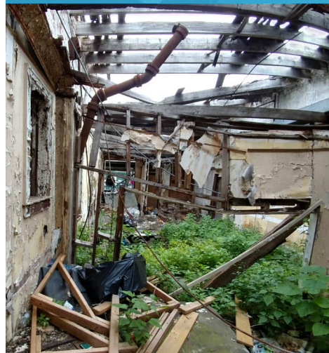
103 King St, Brooklyn. Deteriorated.
